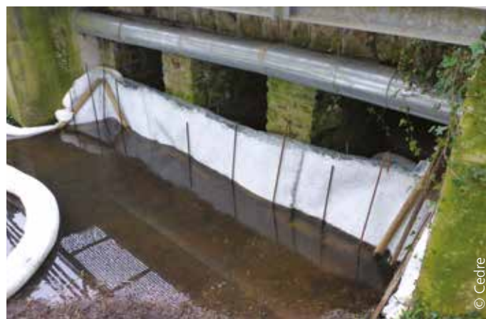
Protection system on the stream downstream of the spill
