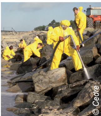
Flushing on riprap
