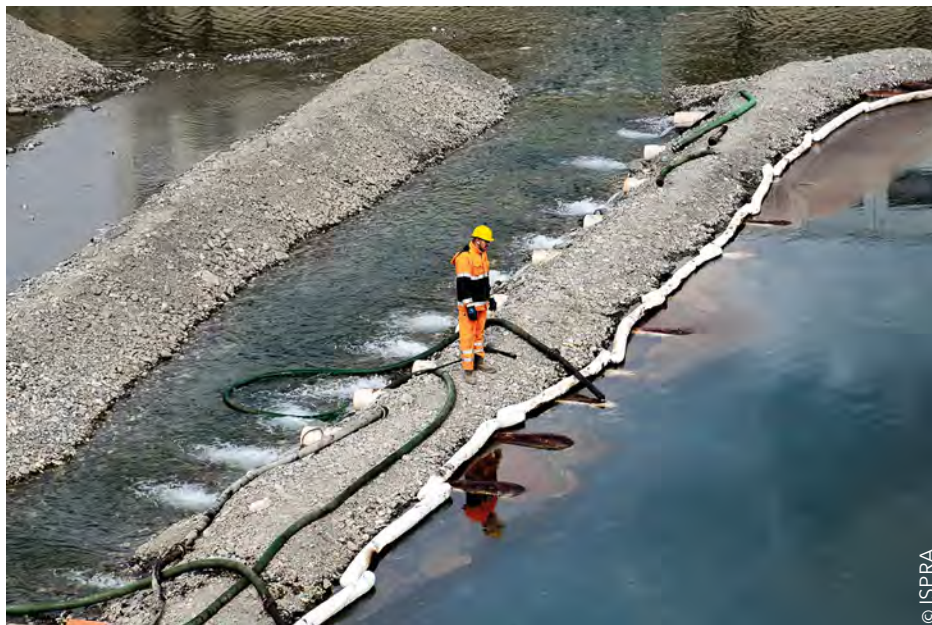
Embankment and sloped pipes used to filter floating pollutant
